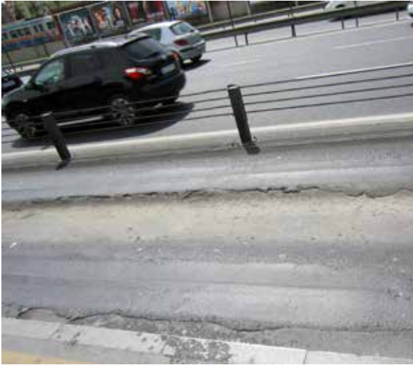
Figure 18 Examples of rutting and similar surface deterioration
