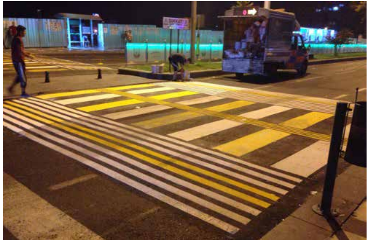
Photo 4 | Construction of the Raised Table Suggested by WRI Turkey Sustainable Cities for the BRT System in Şanlıurfa
